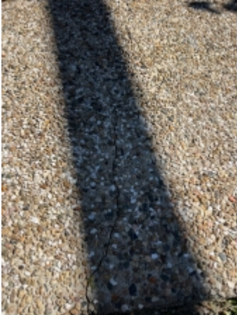
Showing examples of cracking to pathways throughout the property
