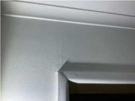
Showing examples of cracking to non-structural elements and paint/finishing defects
