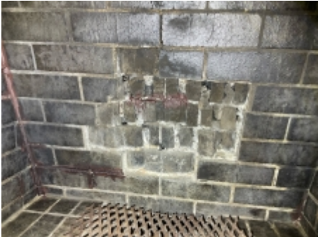
Showing damage to fire place brickwork
