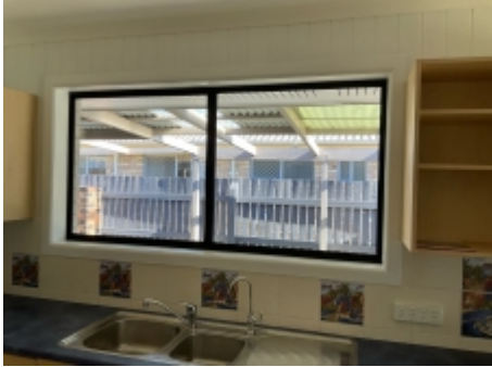
Showing example of windows requires maintenance to operate smoothly
