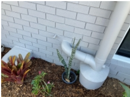
AC unit and Hot water system overflow/s, recommend diverting away from the building or to a suitable drain
