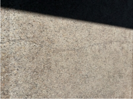
Showing examples of cracking to pathways throughout the property
